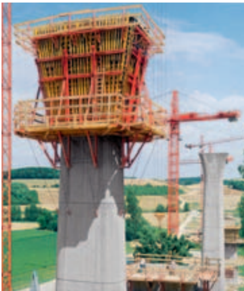
Pier head formwork with climbing scaffold and concreting platforms ready for casting.
