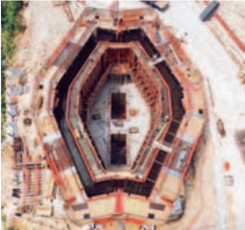
The complicated pier geometry placed high requirements in formwork terms on the construction crew. It was divided into three sections.
