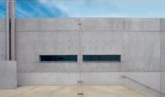
Flexible PERI VARIO girder wall formwork: the formwork joints and fixings along with the arrangement of the tie points were accurately aligned and resulted in a uniform concrete surface.
