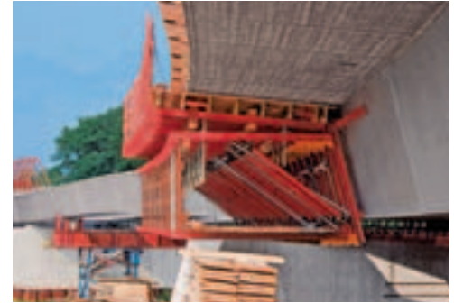
Pre-assembled PERI raised formwork units delivered to the jobsite supported the girder formwork for the superstructure cantilever and safely carried the loads into the steel structure.
