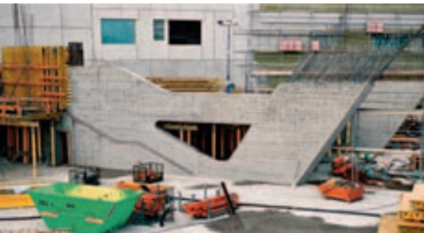
The loads of the upstand beams along with the up to 60 cm thick and 10.00 m high slabs were safely transferred via shoring towers of the MULTIPROP system.
