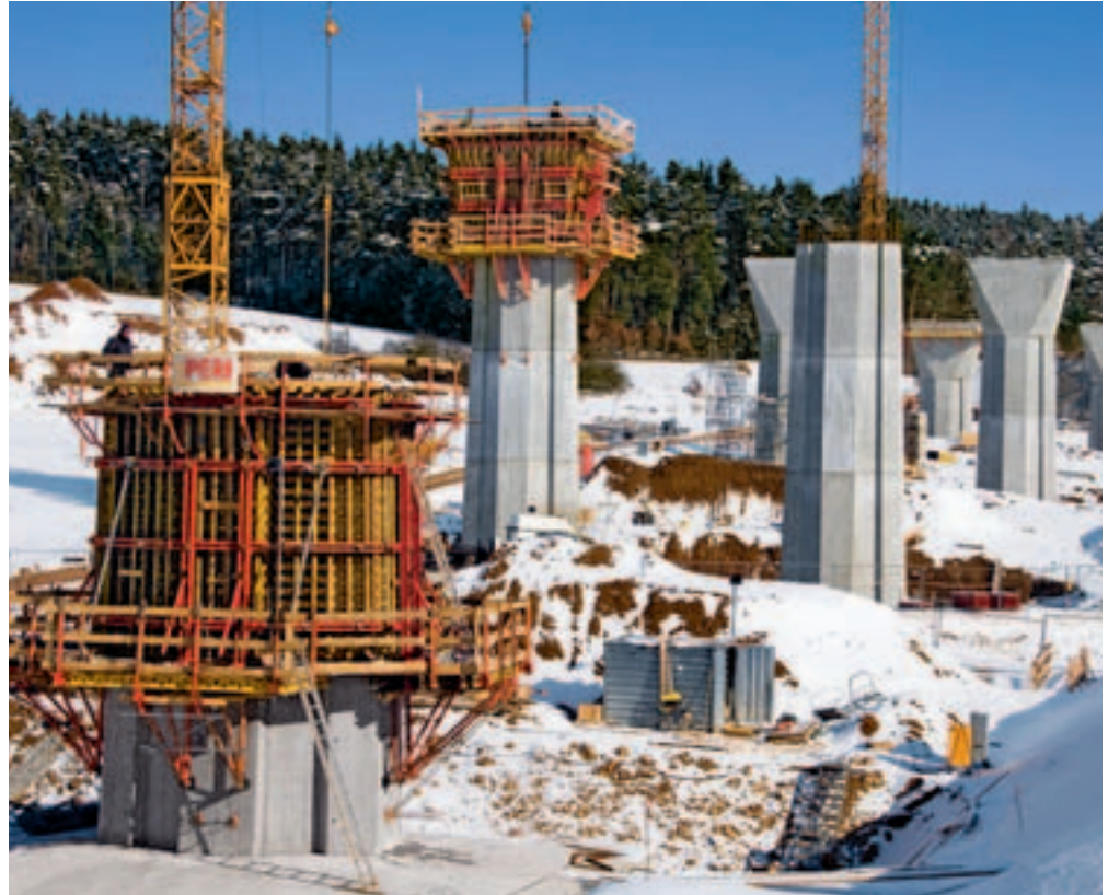
The 515 m long Kulmbachtal Bridge is supported on a total of eight pairs of piers which reach heights of up to 33 m.
