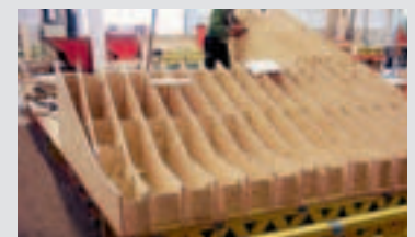
Construction of the 3D formwork units in the PERI assembly hall on the basis of VARIO basic elements.
