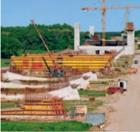
The foreland piers were realised in carefully conducted concreting cycles using VARIO girder wall formwork ...
