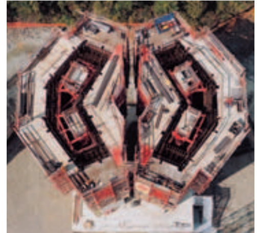
The working platforms formed a platform around the pier cross-section. In the absence of any leading edges, this meant construction crews could work effectively and in complete safety at all heights.
