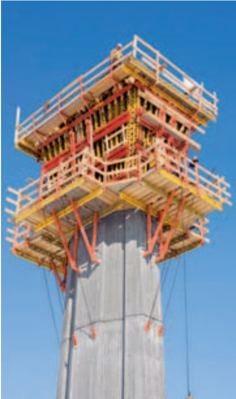
For the pier heads, completely pre-assembled PERI VARIO GT 24 wall formwork elements were delivered to the construction site. The high loads were safely transferred via SKS climbing formwork into the structure.
