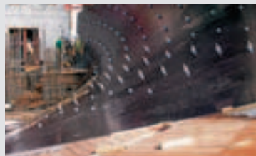
Implementation of the 3D model on the construction site with clearly defined tie positions and formlining joints.
