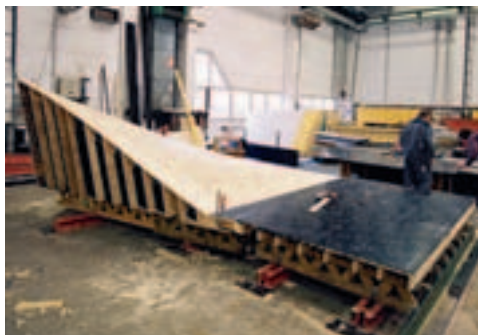
The pre-assembly of the 3D formwork elements in transportable dimensions was carried out by specialists from the PERI assembly service team.
