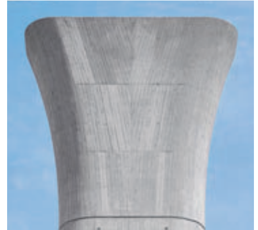
Exact and with the required board structure – one of altogether 16 pier heads after completion.
