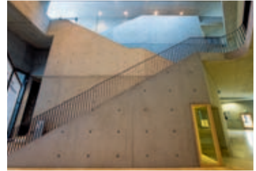
The box-outs for the different window sizes were accurately positioned on the VARIO GT 24 formwork elements according to the construction plans.
