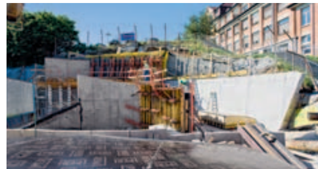
On the construction site, ready-to-use pre-assembled 3D formwork from PERI is accurately positioned and joined together via measuring points.
