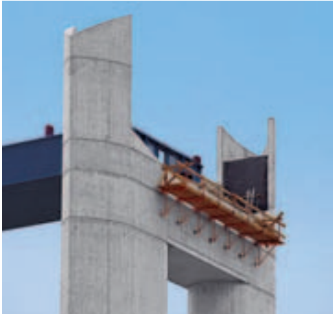
The 126 m high distinctive bridge pylon is constructed in reinforced concrete up to the carriageway, the remainder is in steel.
