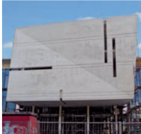
For realisation of the different light apertures and the diagonally-positioned breakline on the facade walls, precision-made prefabricated box-outs were made and doubled up on VARIO elements.
