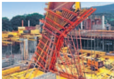
Positioning of the customised formwork from the PERI formwork construction for the inclined column section.
