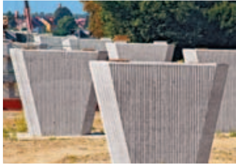
Formwork elements covered with rough-sawn board formwork provided the characteristic surface structure.
