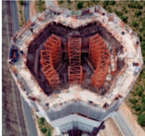
The ACS self-climbing scaffold was used as a working level, for supporting the formwork as well as incremental, crane-independent moving of the formwork.
