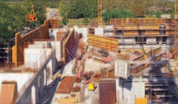
With VARIO GT 24 girder wall formwork for the walls and SKYDECK for the slabs without special surface requirements, the construction team fulfilled the architectural specifications with very high quality.
