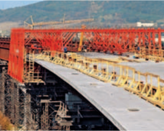
PERI system components for 59 bridge piers in architectural concrete and PERI formwork carriage for the steel composite superstructure
