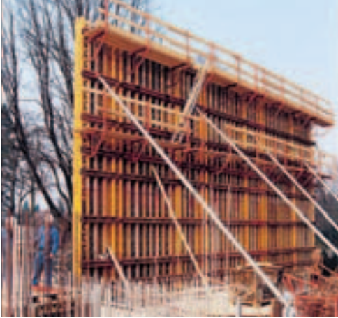
VARIO units 2.50 x 3.00 and 2.50 x 4.80 m were extended to a formwork height of 7.80 m by means of extension splices and later concreted in one pour.
