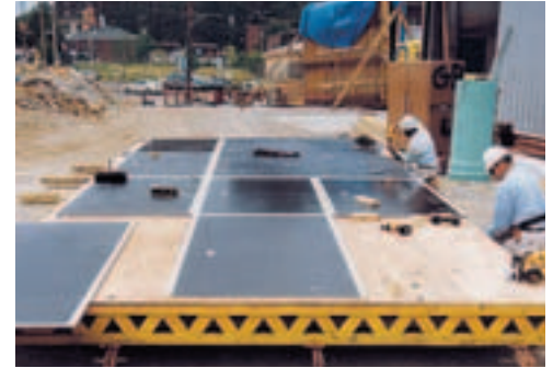
For the best-possible concrete finish, the PERI VARIO elements were fitted with new Fin-Ply formliners after every third concreting phase.
