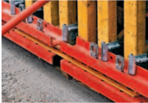
Through the use of the VARIO coupling for architectural concrete, offset-free panel joints could be achieved.
