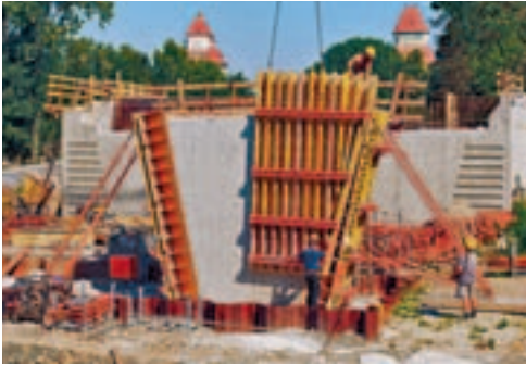
For the twelve pairs of piers in the foreshore area, PERI delivered completely pre-assembled formwork sets on the basis of the VARIO GT 24 girder wall formwork.
