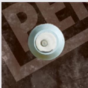
Blind tie on formwork panel
