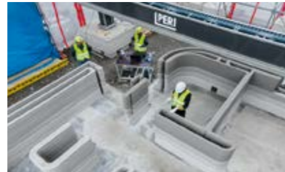
With the BOD2 it is possible to print the inner and outer walls of a building simultaneously.
