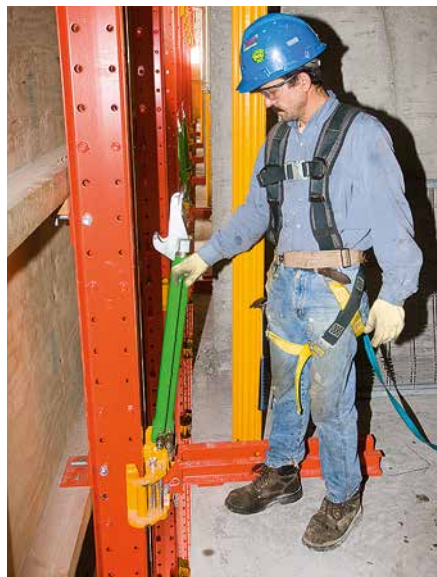
The hydraulic cylinder with its 5 t lifting capacity is positioned on the climbing shoe.
