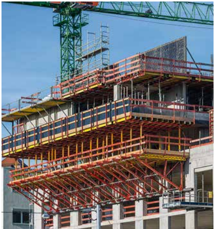
Horizontally positioned Brace Frames could replace high shoring structures for slab cantilevers.
