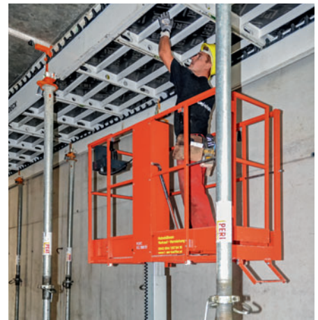
After lowering the dropheads, the central panel is removed first followed by the neighbouring panels.
