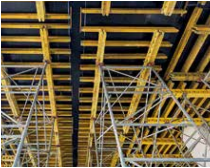
PD 8 Shoring could be quickly and flexibly adapted to suit the different slab heights.
