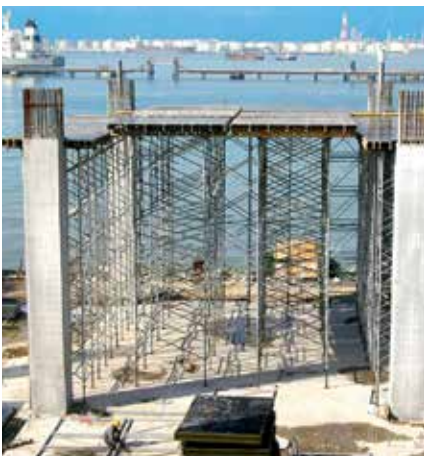
For the construction of this storage facility, 10.50 m high PD 8 Shoring with SRZ Steel Walers as main beams and VT 20 Formwork Girders as cross beams was used.
