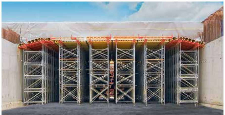
For this tunnel construction, the PD 8 System supports slabs with a slab thickness of up to 1.50 m.
