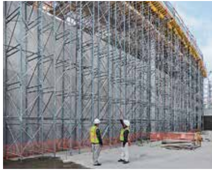
Shoring towers were quickly and easily mounted with only a minimum of personnel whereby the PD 8 Shoring reliably transferred the high loads into the ground.
