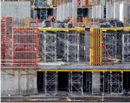
The PD 8 Shoring was the most cost-effective solution for forming the wide-spanded coffered ceilings with the large room heights of over 4 m.
