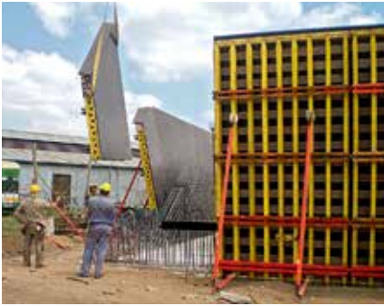
The project-related assembled VARIO formwork units could be used on-site like a system formwork.
