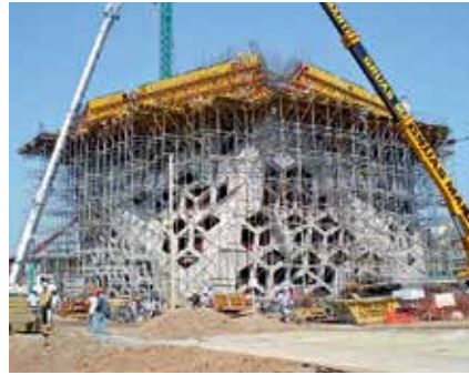
Up to heights of 16 m, PERI UP served as shoring and working scaffold for forming the walls which featured a wide range of inclinations.
