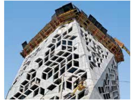
The VARIO formwork on CB 240 climbing brackets climbed heights between 16 m and 45 m.
