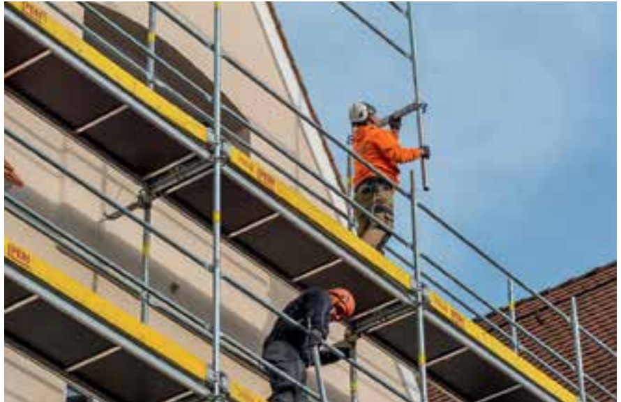
Fall protection without additional components thanks to the systematic assembly procedure with protection provided by the guardrail mounted in advance
